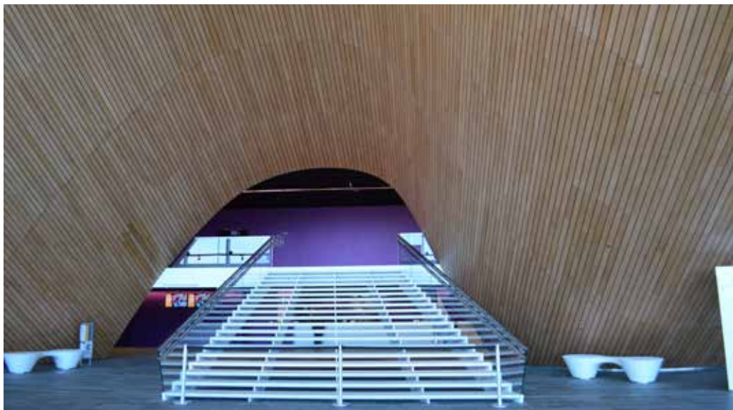
Kilden cultural center in Norway. Billowing oak wall treated with ES/VFR flame retardant coating to B s1 d0.
