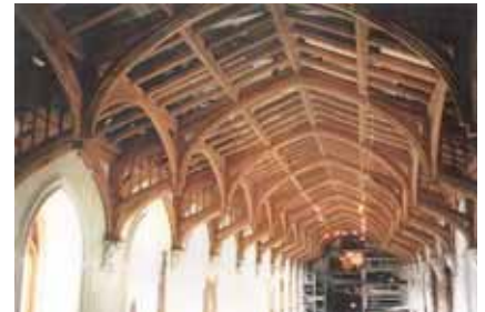
Figure 2.12 'Downsian gothic' trusses at St George's Hall, Windsor Photo: Giles Downes, Siddell Gibson Architects
