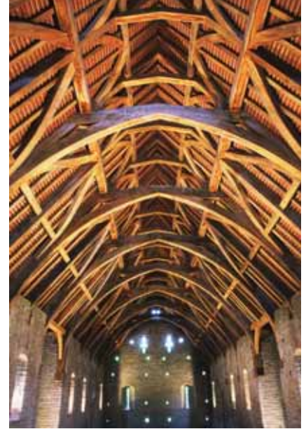
Figure 2.11 (above and left) Pilton Barn, Glastonbury. Reconstruction of roof destroyed by lightning Framing: McCurdy & Co Architect: Caroe and Partners Photos: Wood Awards / McCurdy & Co
