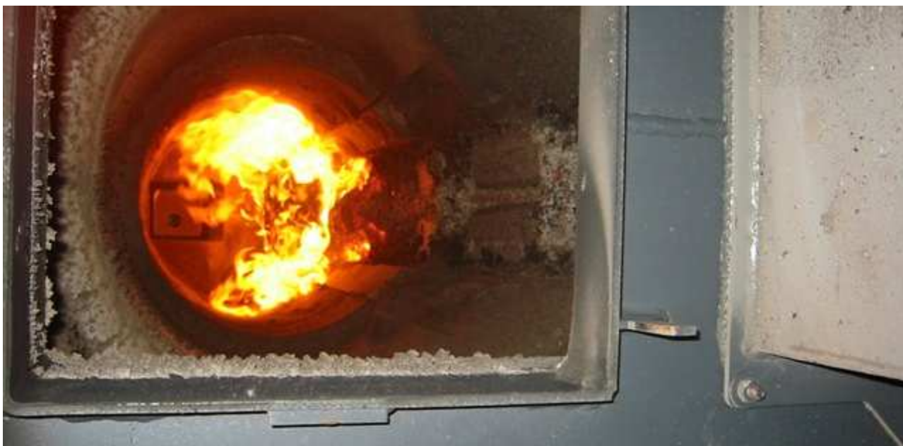
Woody biomass boiler. Photo courtesy of the Biomass Energy Centre
