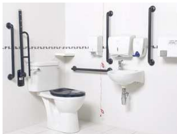
Wall constructions should be capable of taking the fixings necessary for heavy duty grab rails if required.
