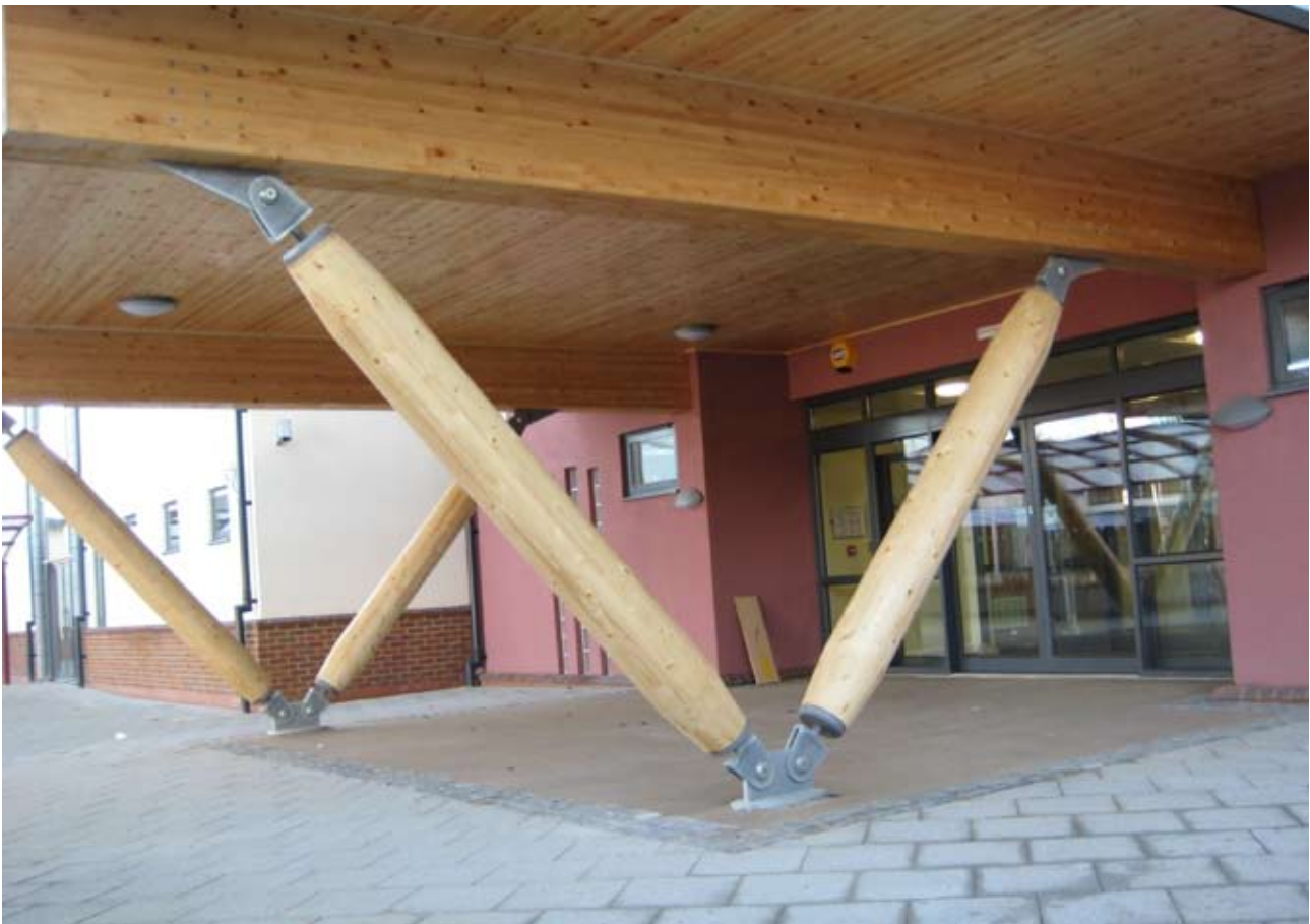
Fig 4. Glulam beams and columns and cross-laminated timber floor at St John Fisher School in Peterborough, Cambridgeshire. designed with EC5. Photo courtesy of Ramboll UK.
