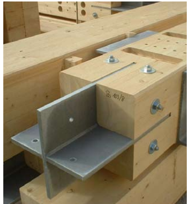
Fig 5. Timber-steel connections at British Geological Survey Office, Keyworth, Nottinghamshire. desogmed with EC5. Photo courtesy of Ramboll UK.
