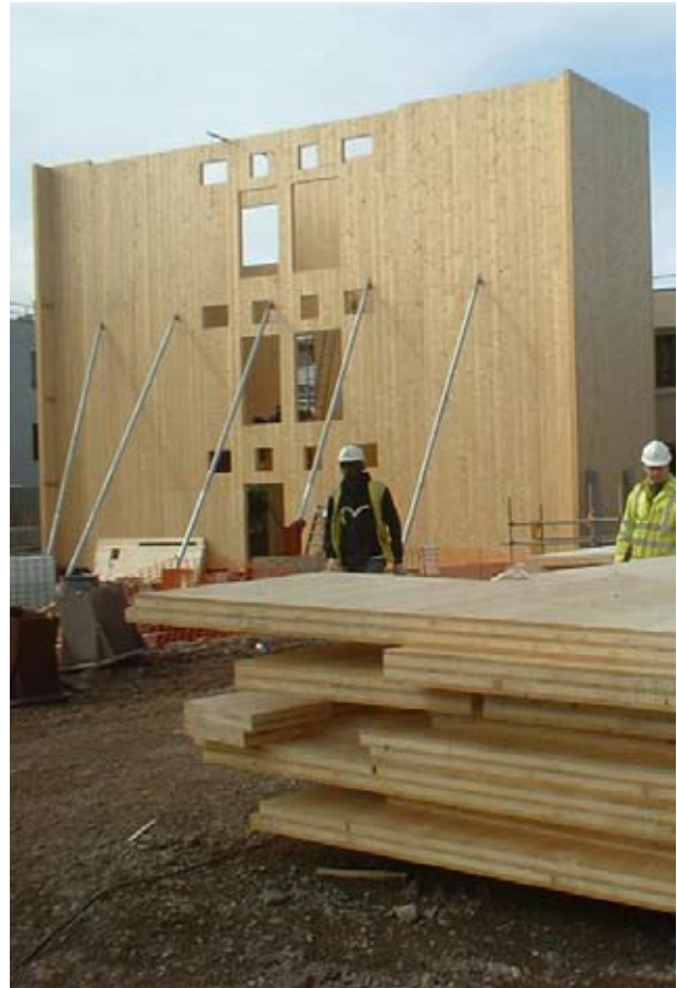
Fig 3. Cross-laminated timber panels at British Geological Survey Office, Keyworth, Nottinghamshire, designed with EC5. Photo courtesy of Ramboll UK.
