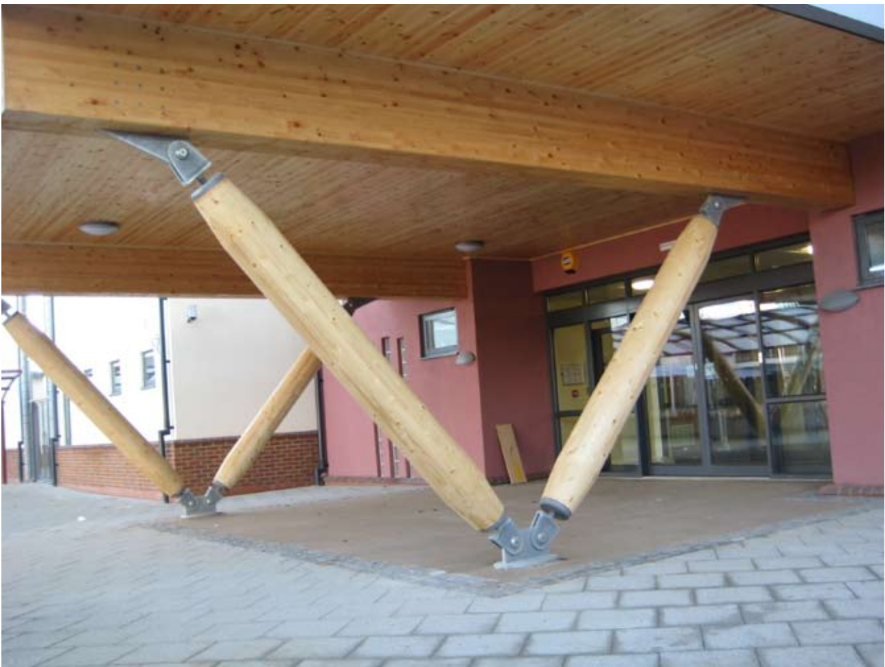
Fig 4. Glulam beams and columns and cross-laminated timber floor at St John Fisher School in Peterborough, Cambridgeshire. designed with EC5. Photo courtesy of the Engineer: Ramboll UK
