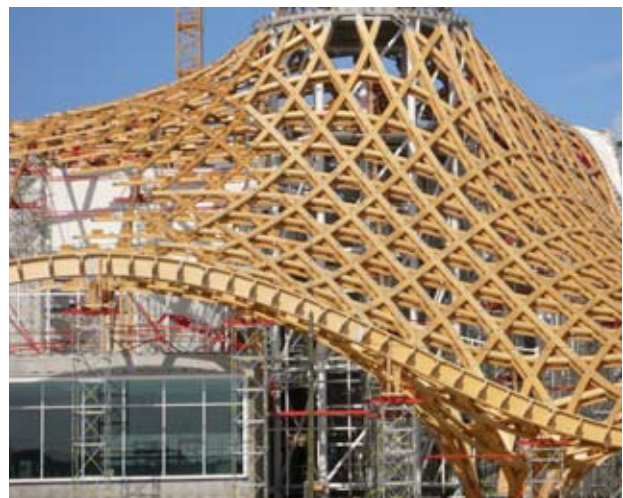
Fig 1. Centre Pompidou-Metz, France, designed with EC5. Engineer: Arup, photo courtesy of the Architect: Shigeru Ban Architects
