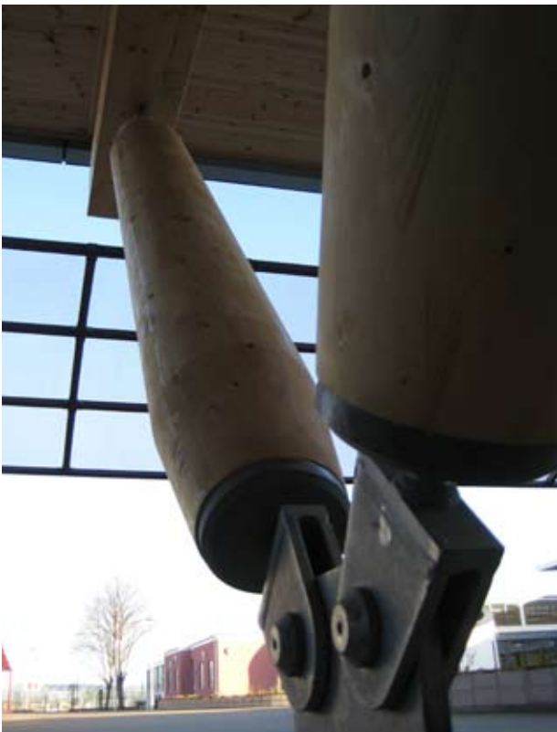
Fig 2. Glulam columns at St John Fisher School in Peterborough, Cambridgeshire, designed with EC5. Photo courtesy of the Engineer: Ramboll UK
