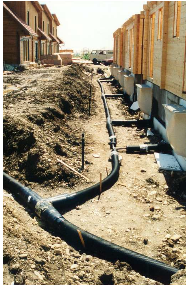
Laying district heating pipes on a new development Photo courtesy of Flexalen Ltd
