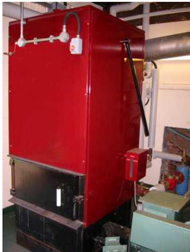
Ashwell wood chip boiler plant.
